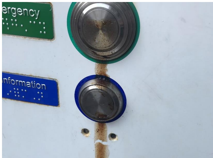
Help points are dirty, damaged or out of service
