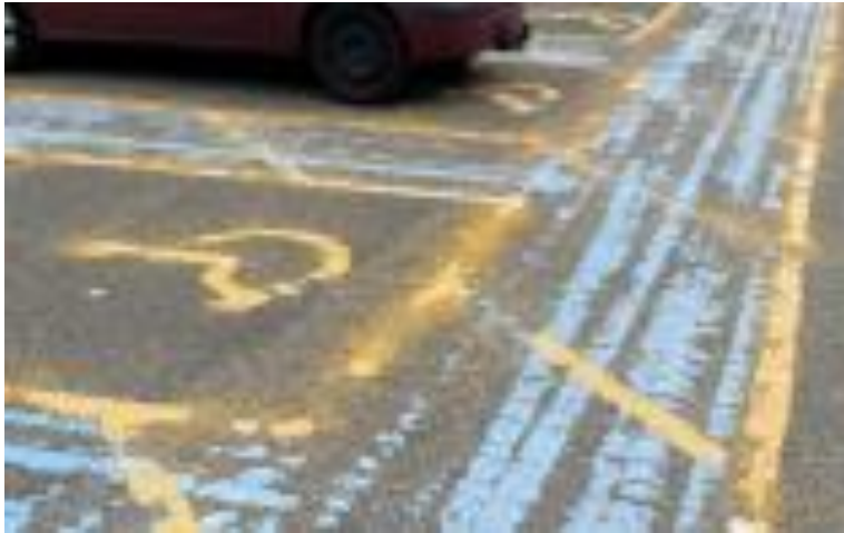
Access to the station from the car park, bus stops, taxi ranks, drop off zones etc. are not very well lit or well maintained
